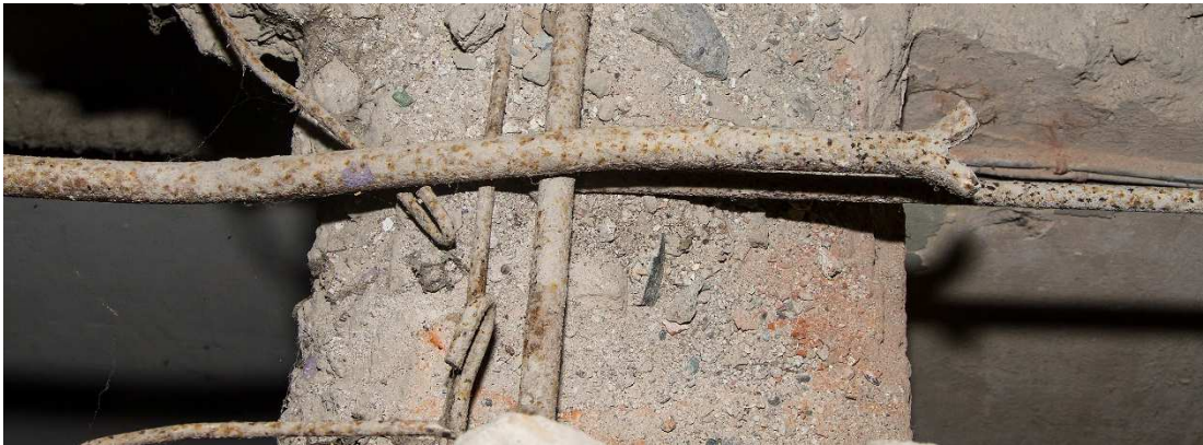
Figure 2. Fish-tail ends and hooks of reinforcing bar of the slab of a villa inside the Villa Gruber park, Genoa, unknown building date, in-between 1900 to 1930.
